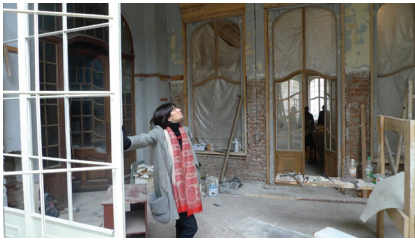
Natasha Lomouri, former director of the Writers' House, stands in the middle of the construction site in the building during its renovation. Photo courtesy of Natasha Lomouri
